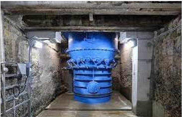
Figure 11: West Nipissing Power Generation Turbine
